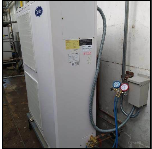
10 TR FLOOR MOUNTED ACU PTC NEP LOGISTICS INC.
