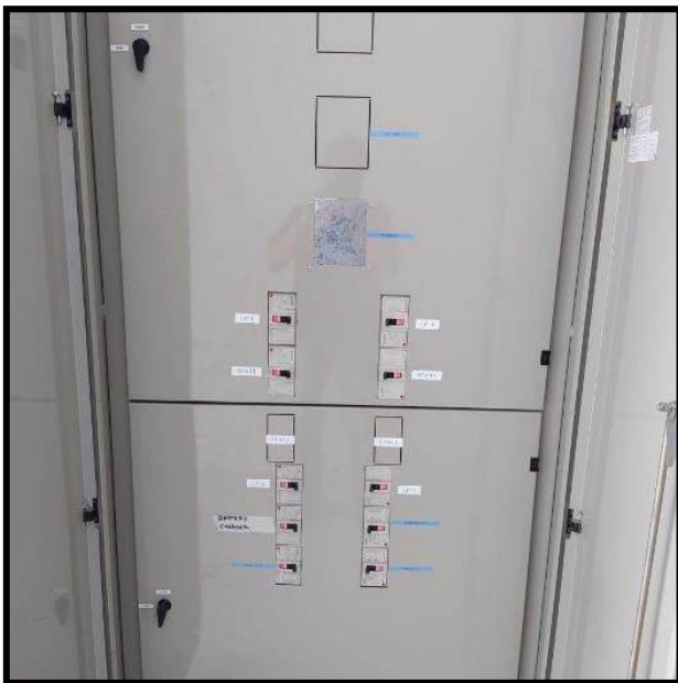
PANEL BOARD SUPPLY & INSTALLATION PTC Nep Logistics Inc.
