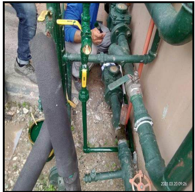
WATER LINE IMI Laguna Technopark Phase 5 Binan, Laguna.
