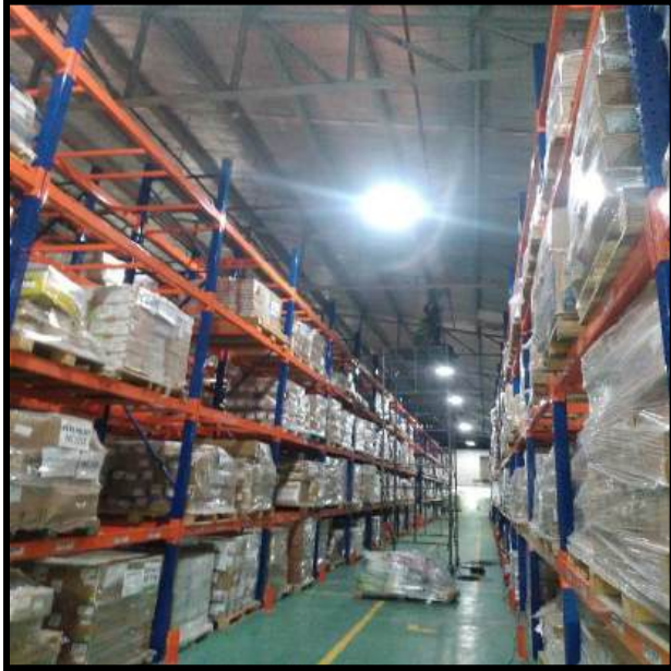
WAREHOUSE HIGHBAY LIGHTINGS Nep Logistics Inc. Epza Rosario, Cavite
