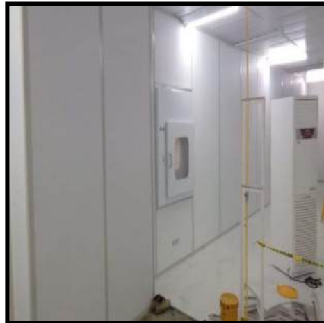
POWERMODULE CLASS 10K & 100K IMI Laguna Technopark Phase 5 Binan, Laguna.
